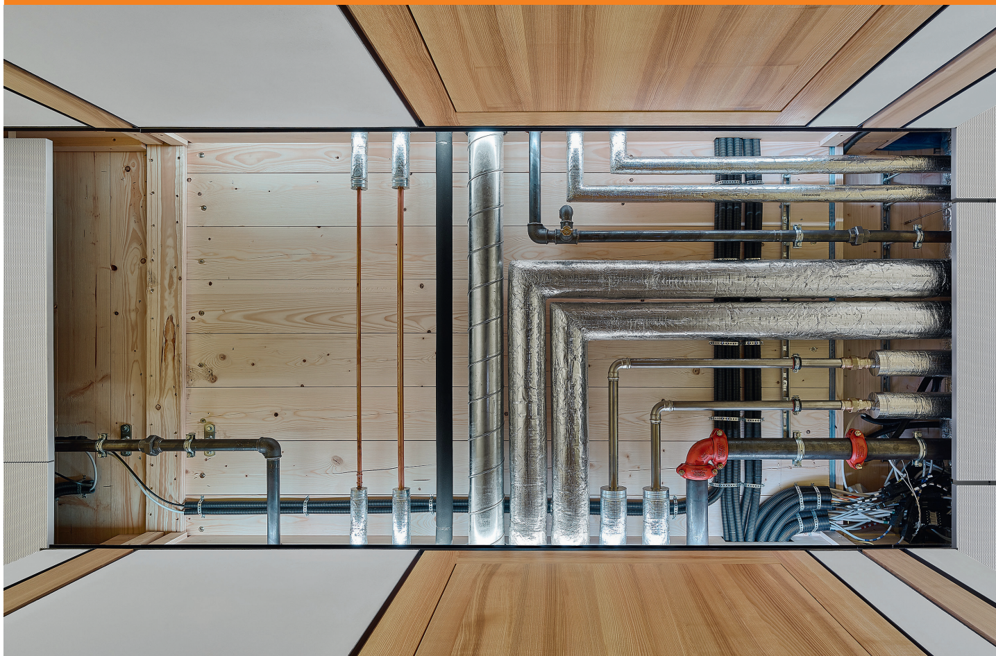
HLK-Infrastruktur in der Nest-Unit Umar in Dübendorf.
